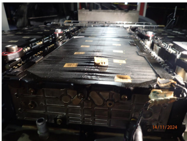
(a) Battery module with thermal damage from E-HK-S.
